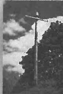
Wireless Antenna On Utility Pole
